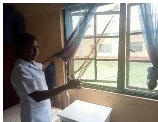
A Nurse holding a torn window mosquito net in the health facility in Idoko community, Etsako East LGA
